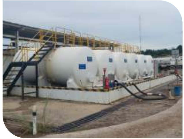
the facility at the emulsion plant fasilitas di emulsion plant
